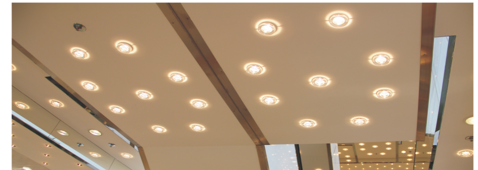
LED spot lighting
